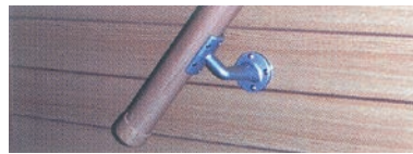
Stairway handrail bracket stop
